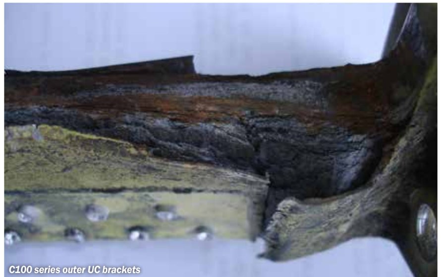
Spar strap showing signs of extreme exfoliation corrosion
